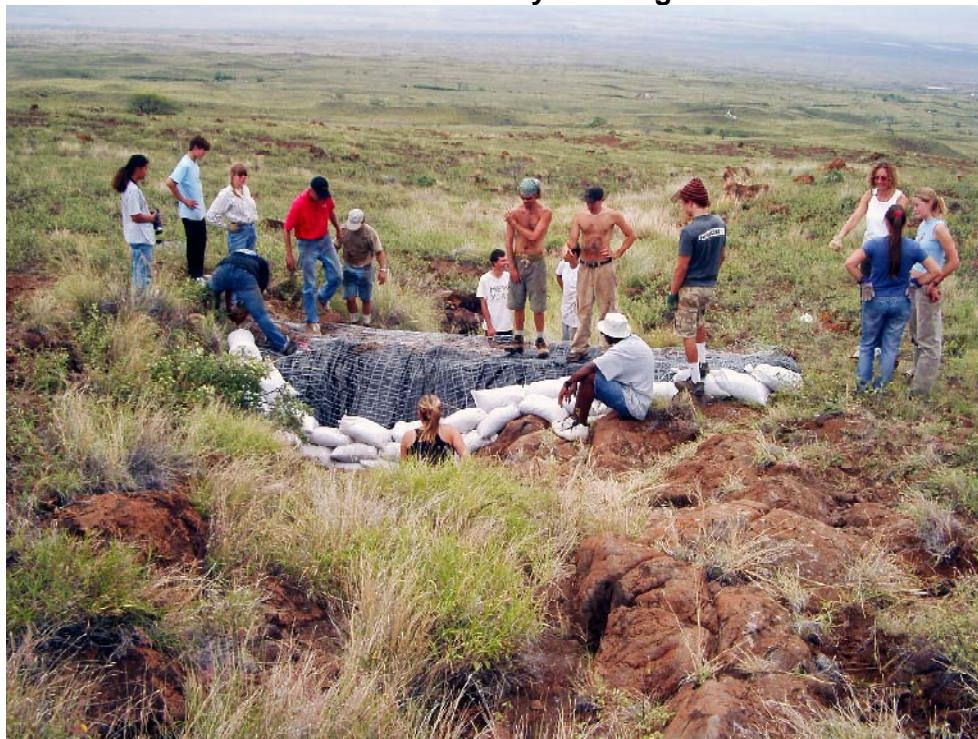
Photo: At the end of the work day building the check dam
