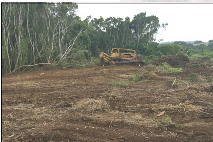
Vegetation clearing, which is an example of grubbing, requires a G&G permit.
