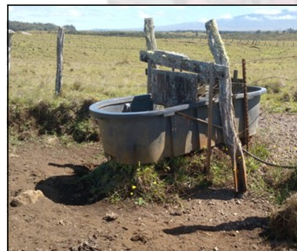
Soil erosion around a trough that can be addressed by moving the trough and adding a heavy use area under the trough.
